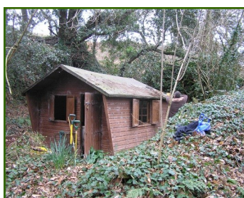
Refurbishment of the shed at Val de la Mare gets underway. The Forgotten Forest Open Days are on June 9th and 10th. Please see back page for more detailed information.
